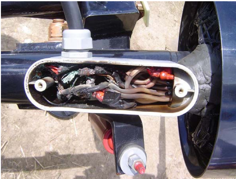
6/16/05 Short in junction box
