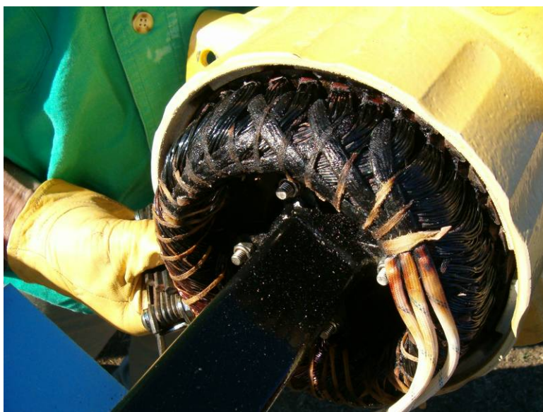
10/4/04 Hurricane damage, burned alternator
